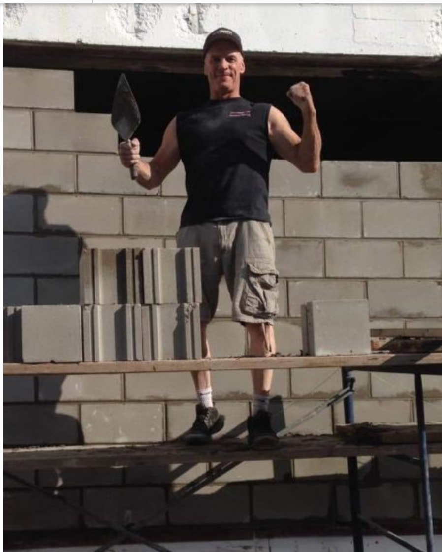
Portland Boxing Club volunteer Jon Webster bricking over a former window opening at the Portland Boxing Club building during August 2019.
